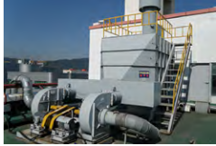
Activated carbon adsorption facility
